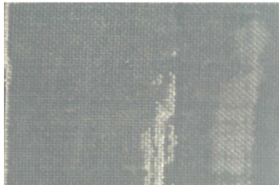
Figure 4. Impact induced damage
