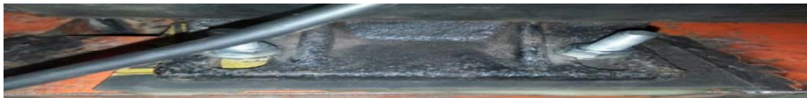
Figure 14. Composite material under the motor base.
