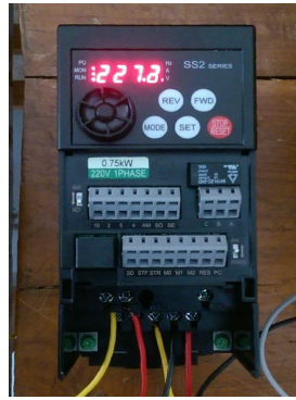
(e) Inverter Converter Set-1
