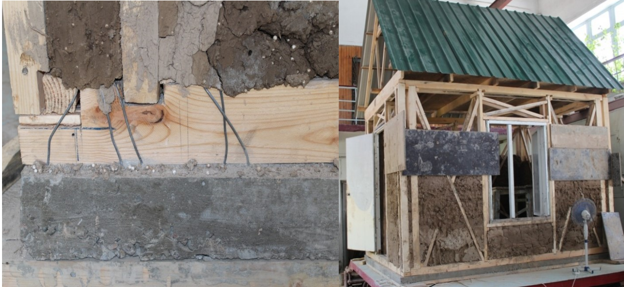
Fig 3. The process of construction of a model house of wooden frame "synch"
