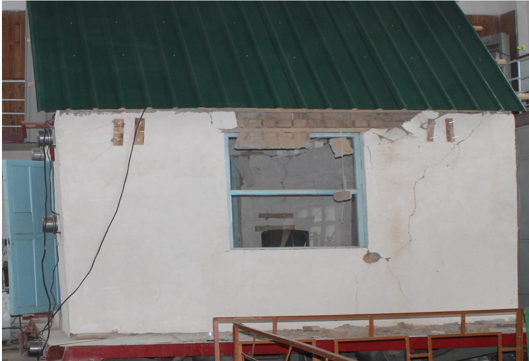
Fig2. General view of the model of the house, made of brick raw, after the experiment
