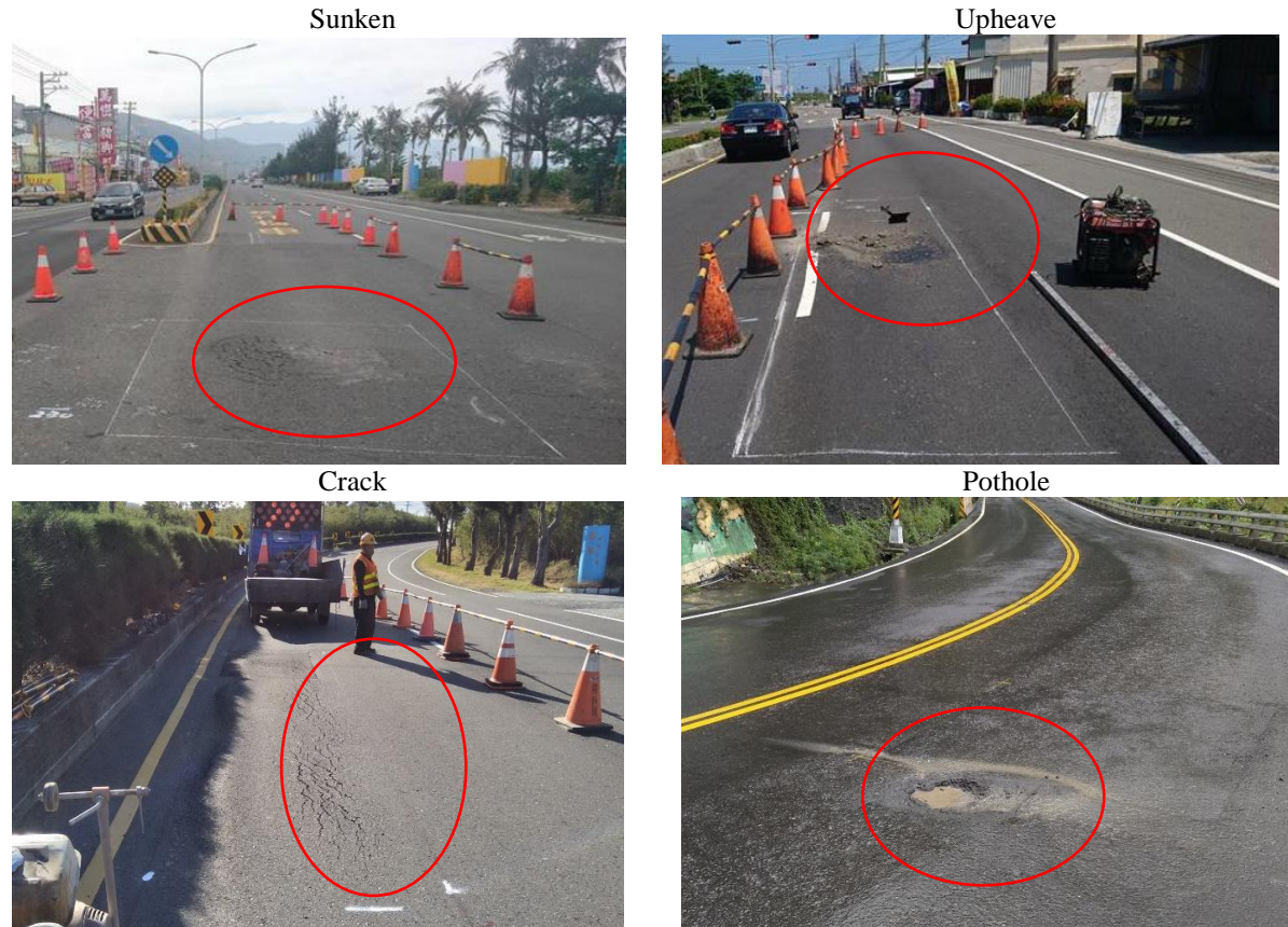
Figure 2 Examples of asphalt pavement damage along the road section studied herein.
